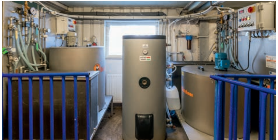
CulinaCup feed kitchen with two mixing tanks
