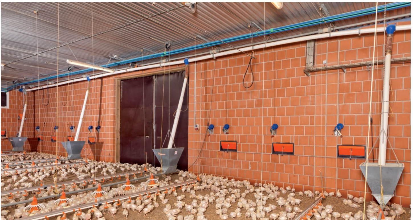
Use of cable winches for optimum height adjustment of the drinker lines in relation with the birds' age
