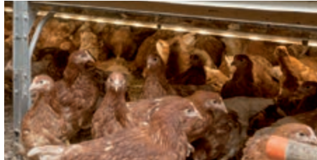
FlexLED to light the litter area below the system
