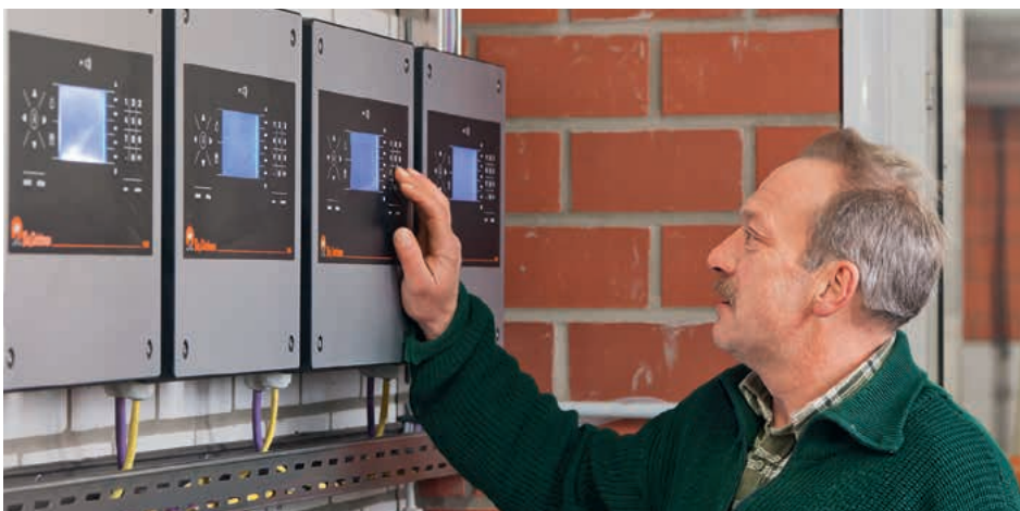
Each sorting scale TriSortpro is managed by a control unit, in this case installed in the service room
