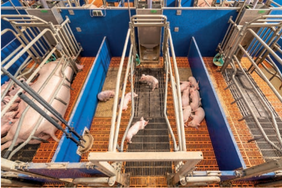
Flooring system with plastic slats and integrated heating plates for the piglets and cool cast iron slats for the sow
