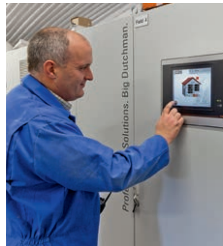
Additional touch screen in the control cabinet
