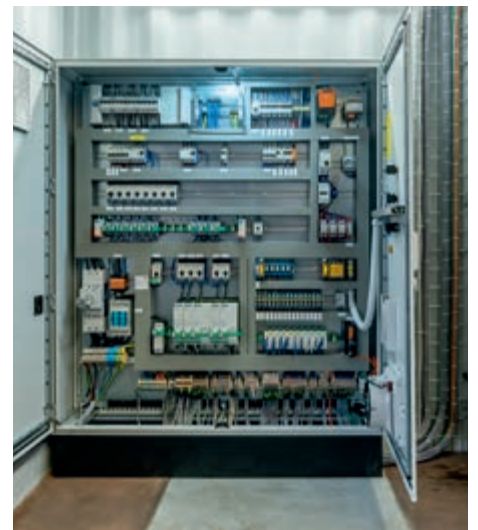
Control cabinet integrated into the container
