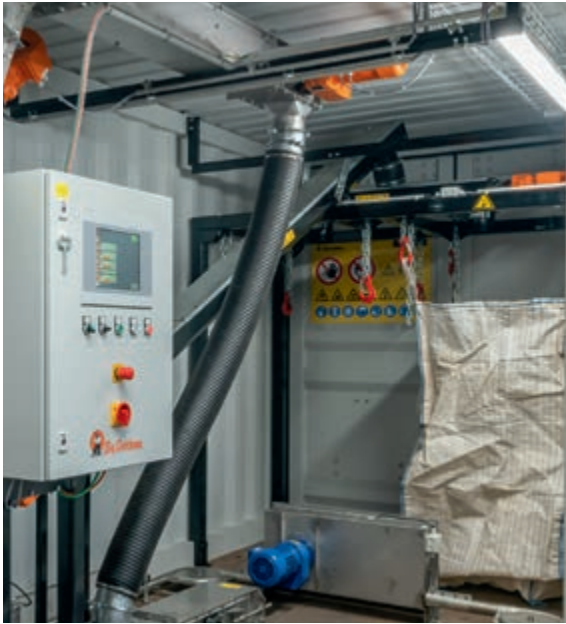
View of the BigBag bagging unit
