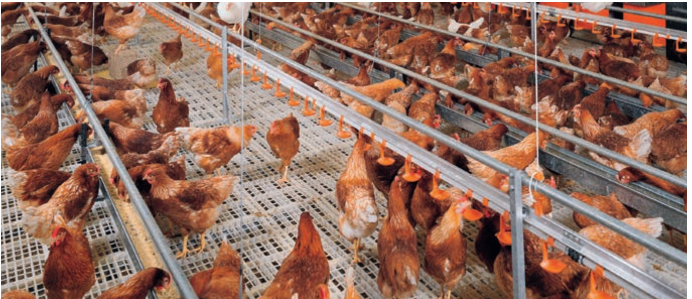
Nipple drinkers and chain feeding system, installed in both suspended and standing position
